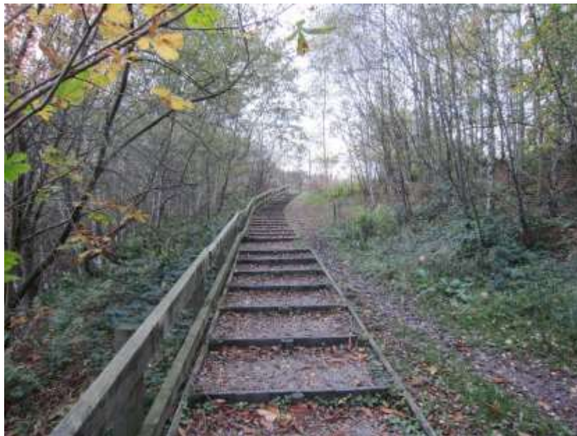
Most of the vegetation has been moved from the steps.
